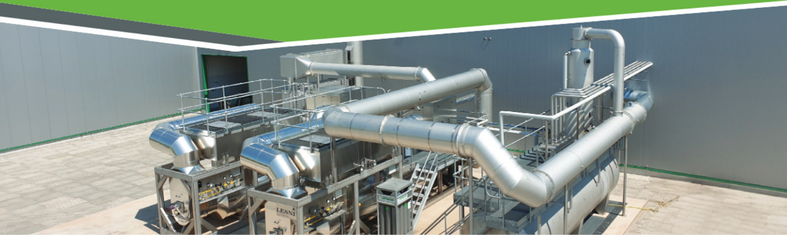
Figure 1. LESNI EO CAP, which Picarro technology shows abates EtO emissions well below the new NESHAP requirements proposed by the US EPA.
